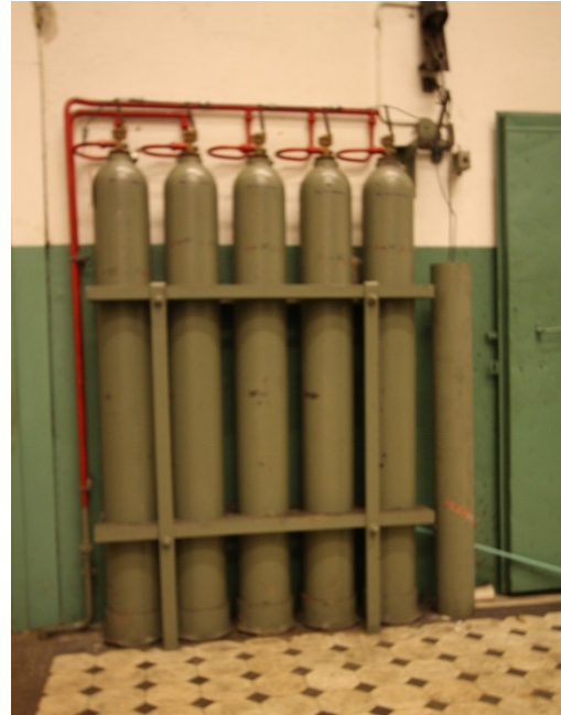
CO2-flasker for brannslukking.
