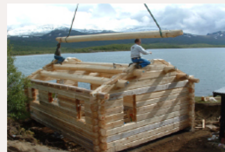
Nowadays the majority of new log buildings are holiday cabins. Log cabins are manufactured in large industrial buildings and brought on site and erected quickly using modern technology. Here you can see the ridgepole being installed. Photograph: Tor Henning Evensen
