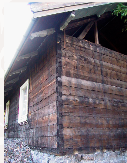
Log house under restoration. The panel has been taken down temporarily. Note that the wooden apex is not made of logs. This is a commonly-used method.
