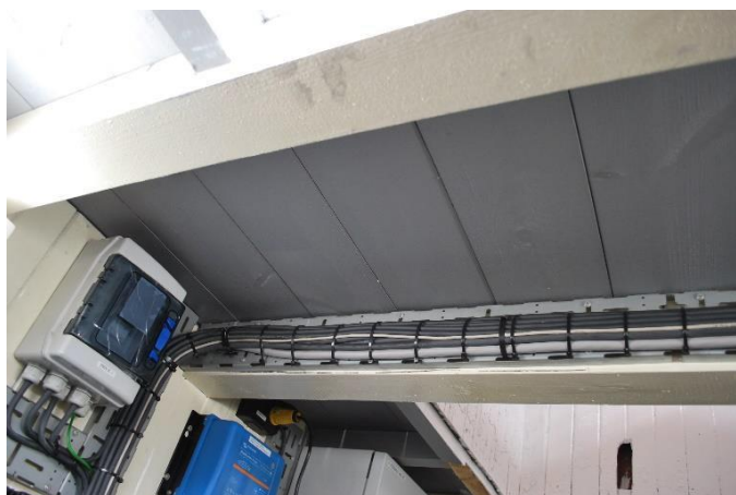
EI.kabler – himling skylight/nedgangsskappe.
