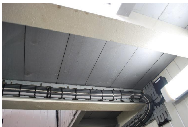
EI-kabler langs bjelker i himling maskinromcasing.
